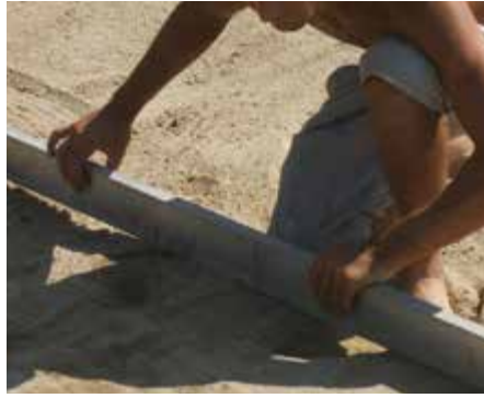
② LAYING BASE Lay the sand bedding (at least 10 cm) of volcanic sand or silicium sand enriched with fertilizers.
