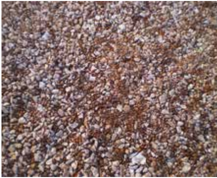
① DRAINING BACKGROUND Excavation and creation of a draining layer made of gravel or lapillus (minimum 15-20 cm).
