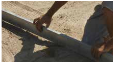
② LAYING BED Creation of SALVAVERDE Geoplast laying surface formed by 3/4 cm of volcanic sands mixture (enriched with soil and fertilizers), grain size 0-5 mm laid out and well struck in order to reach a perfect leveling.
