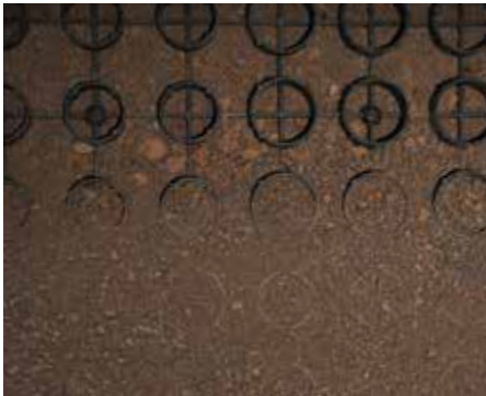
④ FILLING Grid covering with the same sands of the sand bedding up to the edge.
